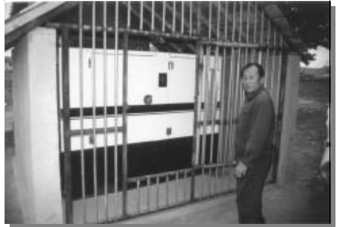
Newly installed generator at the Haeju TB Hospital
